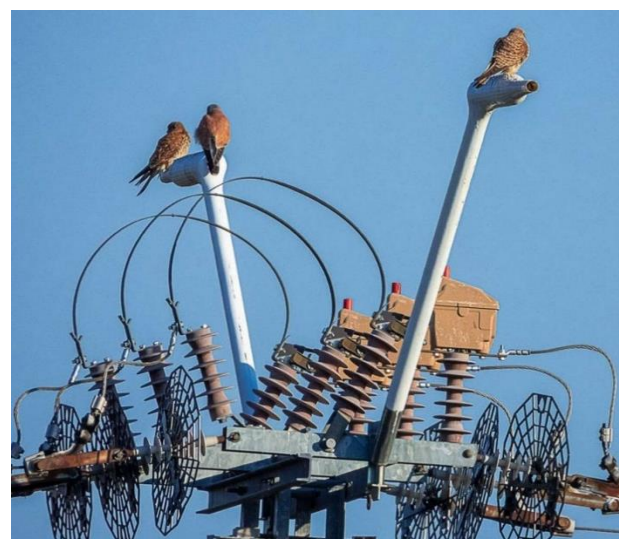
Fig. 4. Safeguarding by installing perches and bird discouragers.
