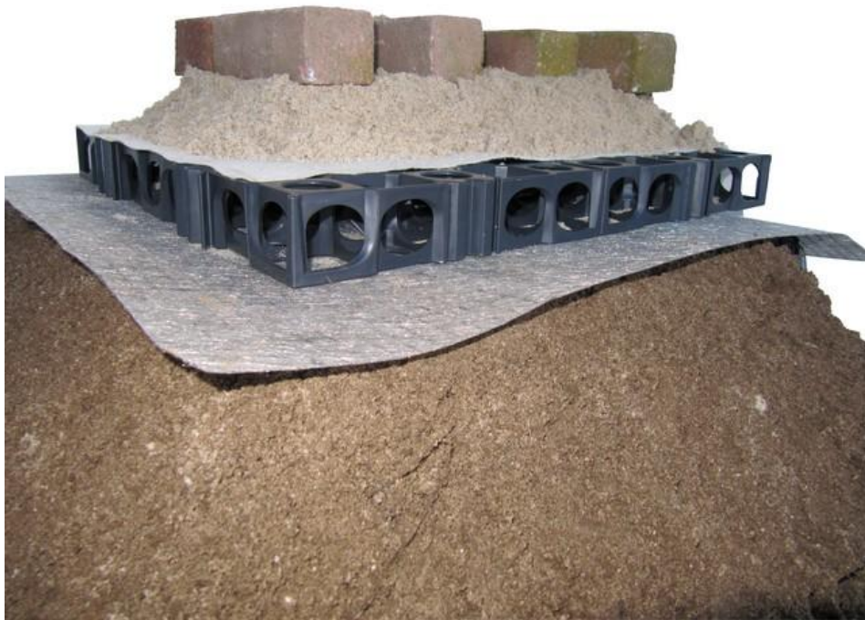
Fig. 3. Laying of ground flooring with a root bridge module (sandwich panel). ( https://www.greenmax.eu/nl/sandwichpanel74 )
